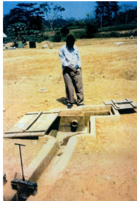
Fig. 3a: influent channel
