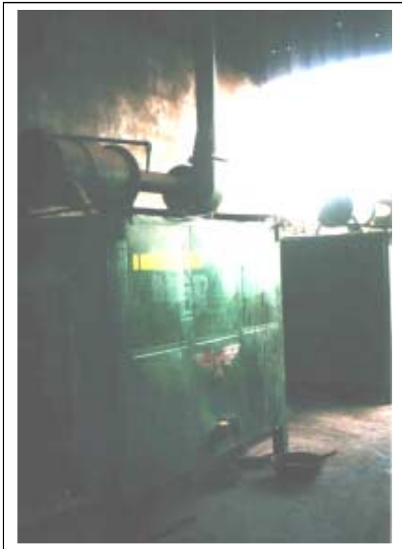
Pic.11: Chamber furnace for the carbonisation of briquettes from agricultural residues in Mali /2/
